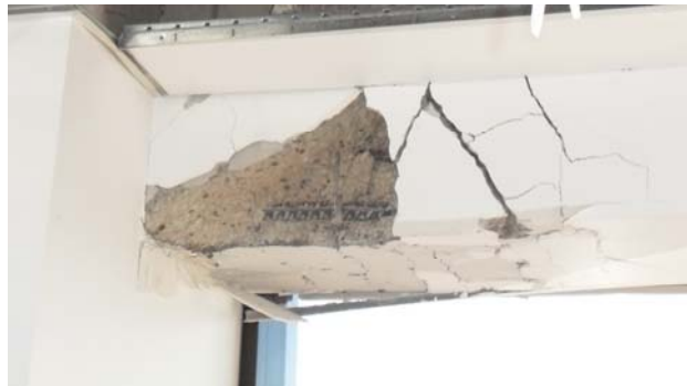
Figure 1: An energy absorbing (ductile) beam hinge in a reinforced concrete building after an earthquake. As these ductile elements yield they absorb energy without loss of strength that would lead to collapse of the building. While some of the cover has fallen off, none of the reinforcing has broken, and the concrete inside the reinforcing cage is intact, so this beam can still carry load.
